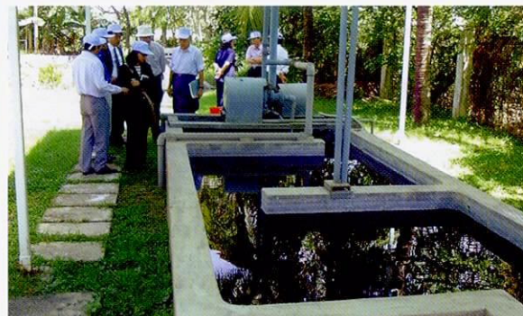
Wastewater treatment equipment at pesticide plant
