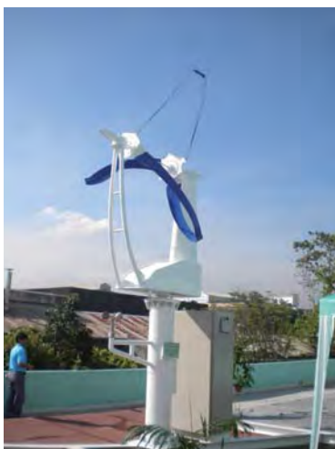
A small wind turbine installed on the roof of the Department of Science and Technology
